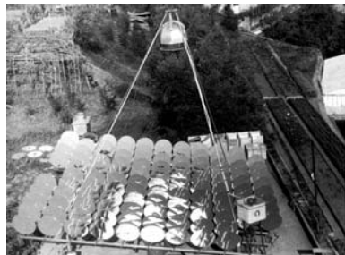
Fig. 7: The first point-shaped solar boiler, installed at Sant'Ilario di Nervi in 1965 (Photo Ansaldo Review N. 11/81)
